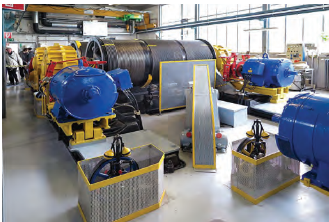
The massive cable drums and winding gear for the vehicle lifts in the southern Old Elbe Tunnel shaft. The equipment is meticulously maintained including the traditional governors in the foreground
